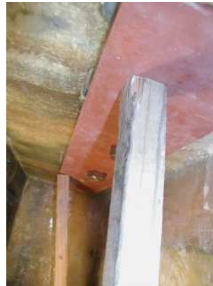
ARG installation surface (bottom view)
