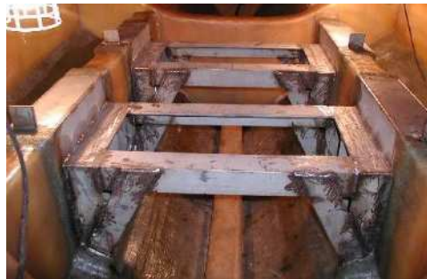
Example of setting up iron trestle for FRP ship Figure 3-2 Reinforcement of ship
